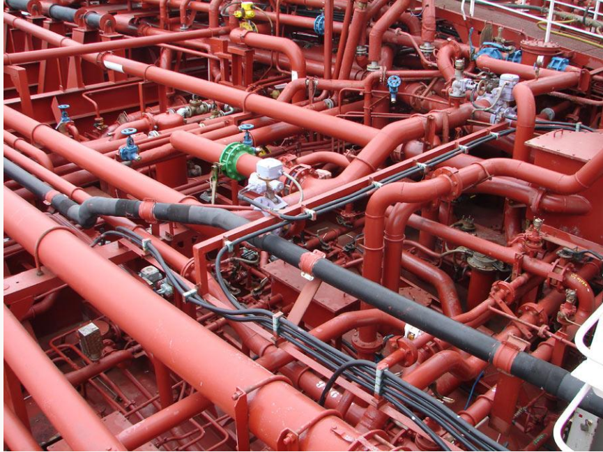
Piping system on a chemical tanker, by Hervé Cozanet, CC BY-SA
